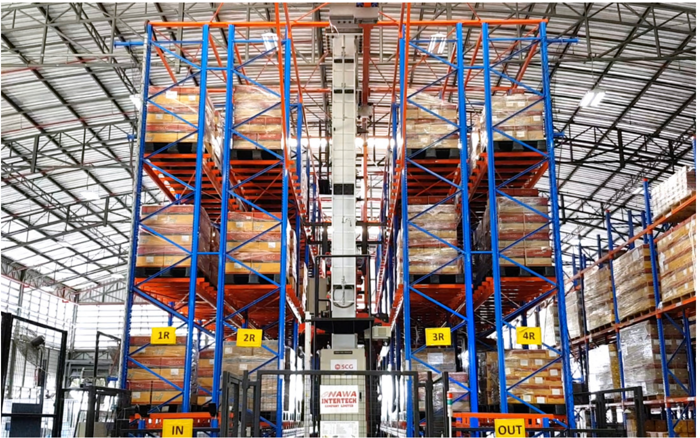
Automated Storage and Retrieval System (ASRS)
